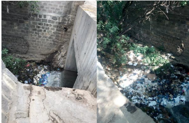
Figure 9. Collection of rubbish downstream of the existing culvert
